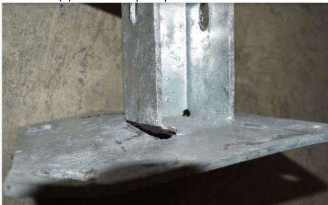
(c) Ductile baseplate fracture at welding
