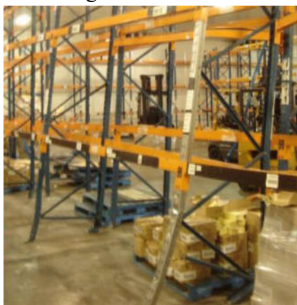
Figure 2: Cross-aisle direction failure by column buckling [3]
