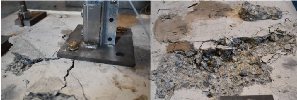
Figure 11: Rigid baseplate anchor bolt pulled out
