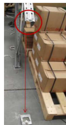
Figure 4: Fracture of baseplate connection [4]
