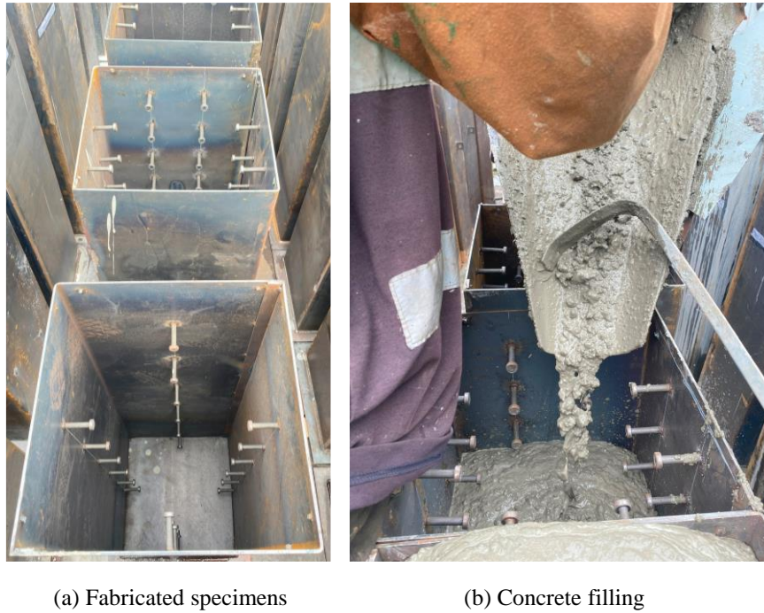
Figure 1: (a) Steel tubes fabricated with welded shear connectors; (b) filling of concrete.
