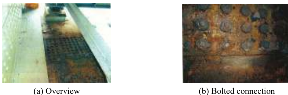
Figure 1: Corroded bolted connection.
